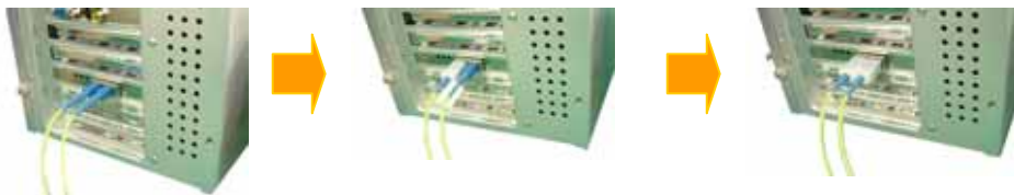
Plug connectors. completed.
