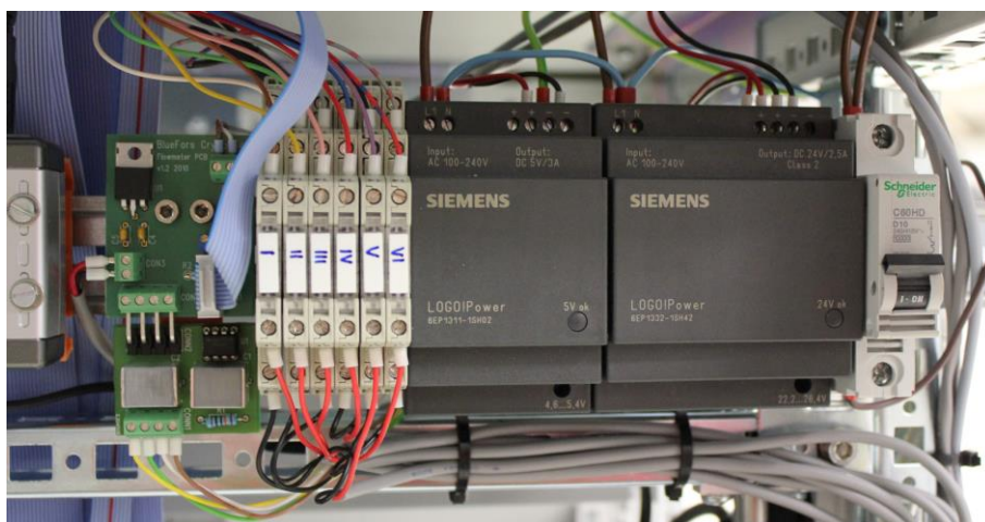
Location of the flow-meter PCB inside the control unit
