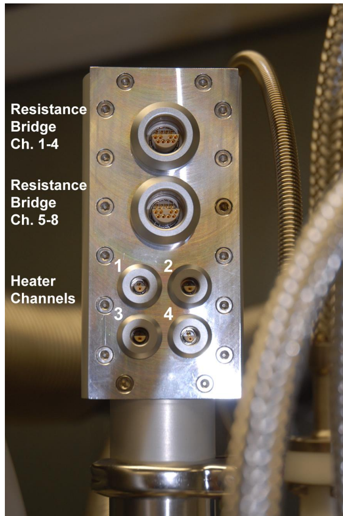
Figure 15. DR wiring connector box.
