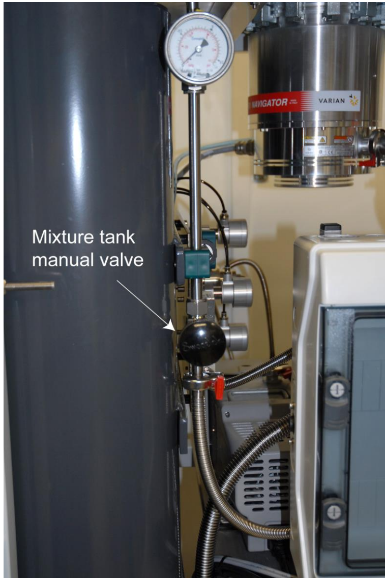
Figure 18. Mixture tank manual valve.
