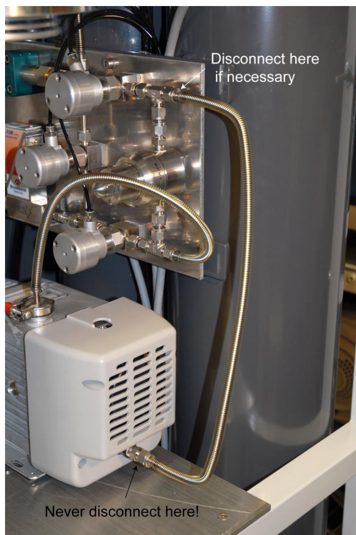
Figure 24. Compressor service warning.
