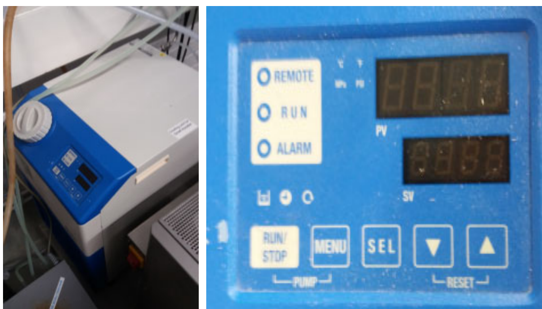
Image 3 - Cooling unit / control panel
