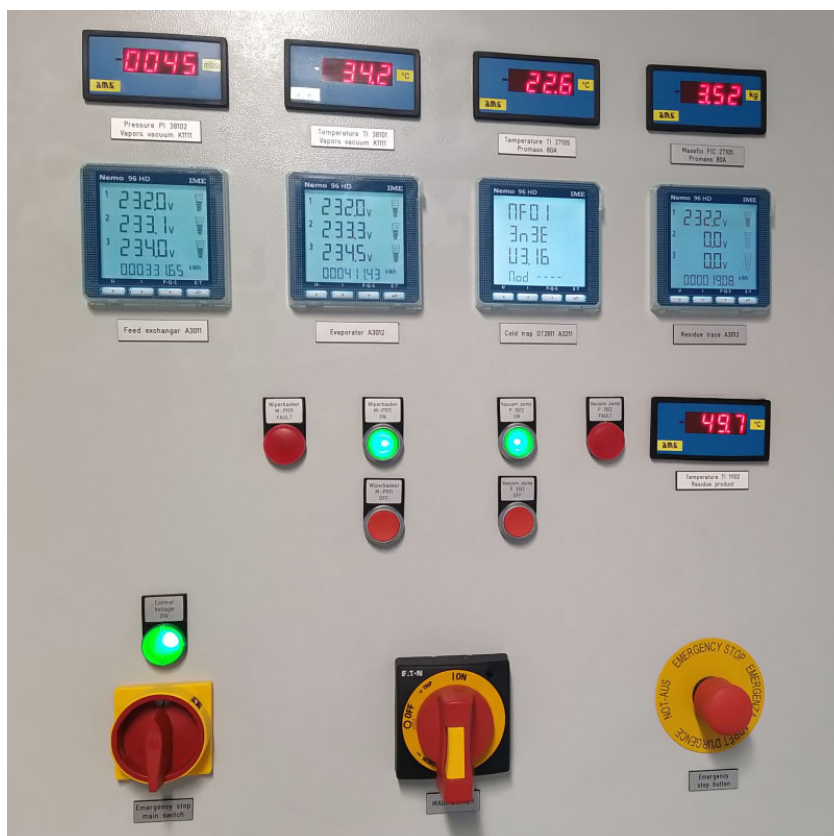
Image 1 - Main Control Panel
