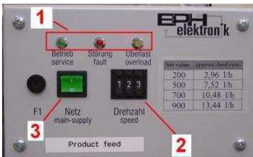
Image 13 – Feed Pump Console
