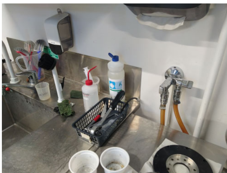
Image 6 - Cooling Water Tap
