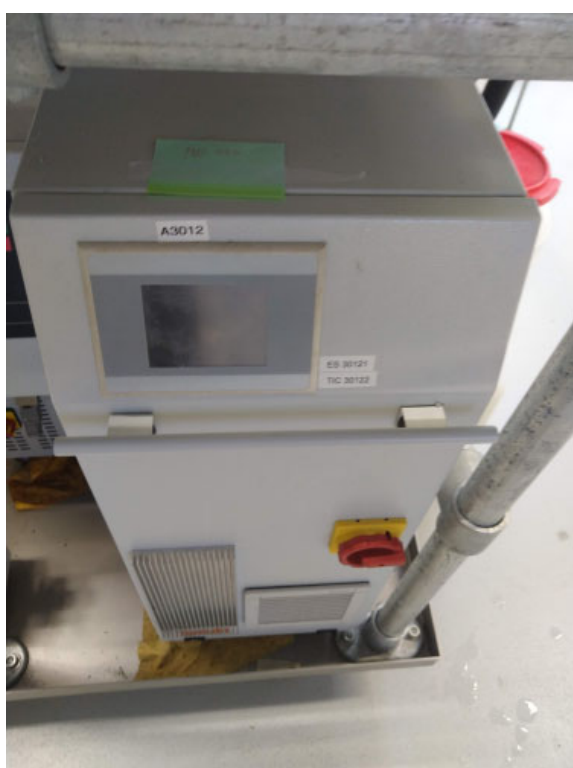
Image 8- Heating Unit A3012
