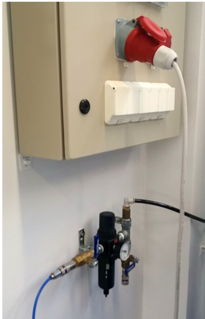
Image 3- Power and pressured air connected, air valve closed
